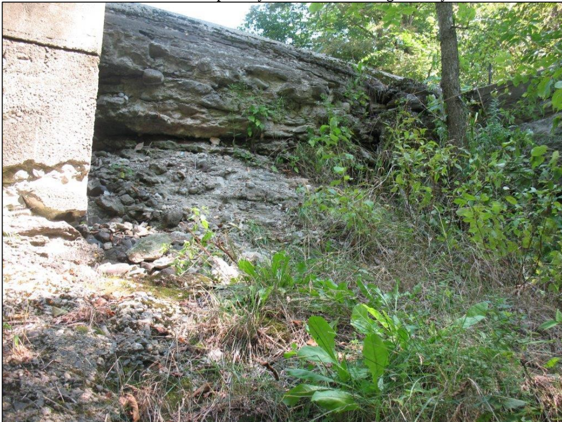
Photo 8. Left Nonoverflow: Deteriorated Downstream Face and Backfill. Note Vegetation and Large Tree.
