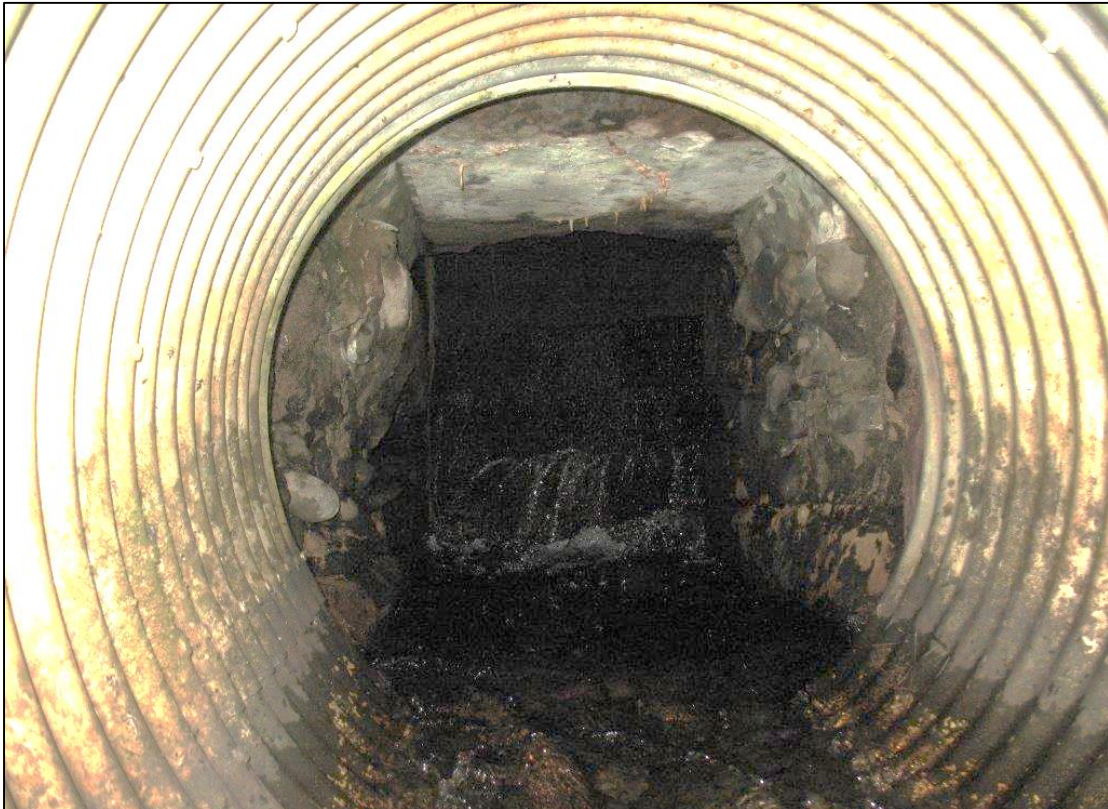
Photo 14. Leaking Gate of Left Outlet.
