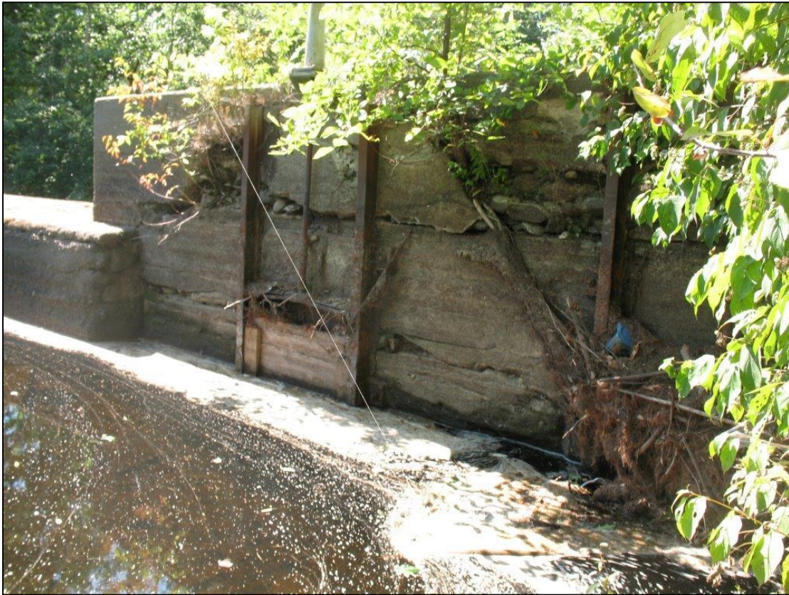
Photo 13. Right Nonoverflow: Left Outlet Timber Gate and Deteriorated Upstream Face.
