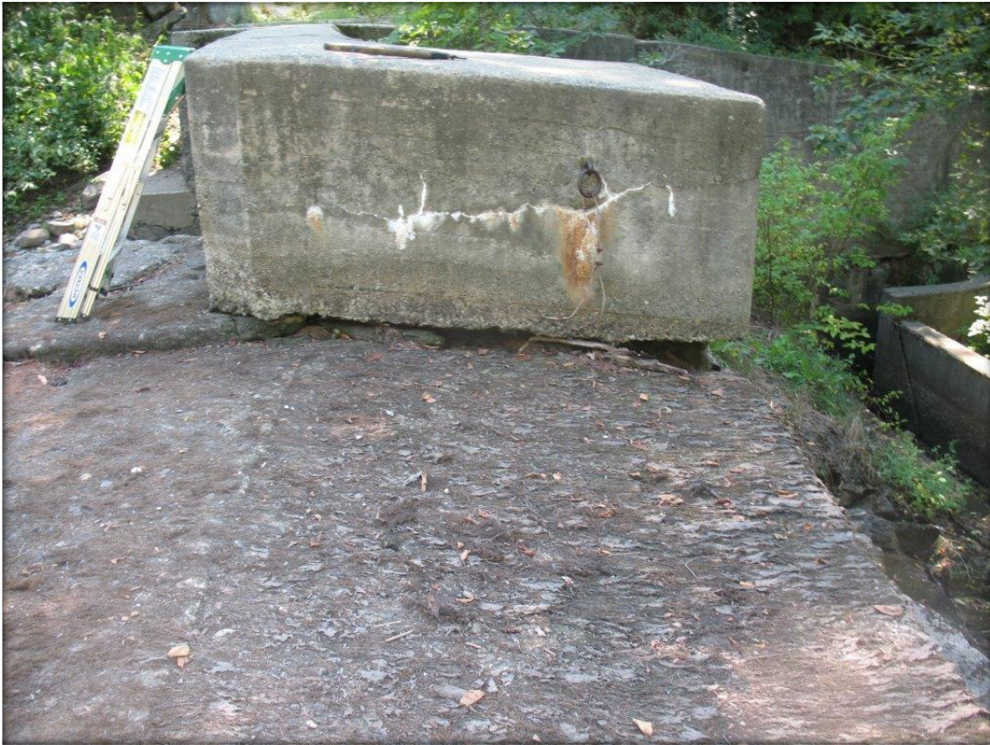
Photo 5. Left Spillway Pier Undermined Base.
