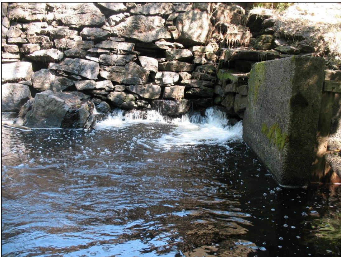
Photo 4. Extensive Leakage at Spillway Toe near Fishway.
