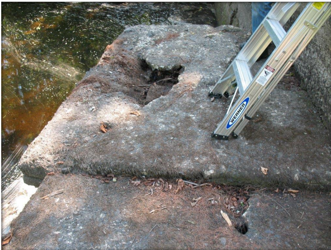
Photo 2. Large Cavity in Spillway Crest Extension at Left Nonoverflow Structure.
