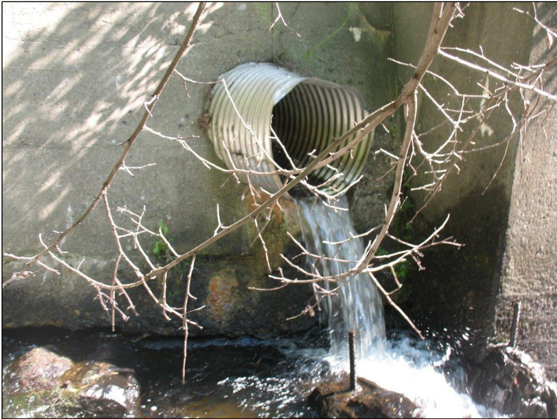
Photo 15. Leakage Discharge from Left Outlet Culvert.
