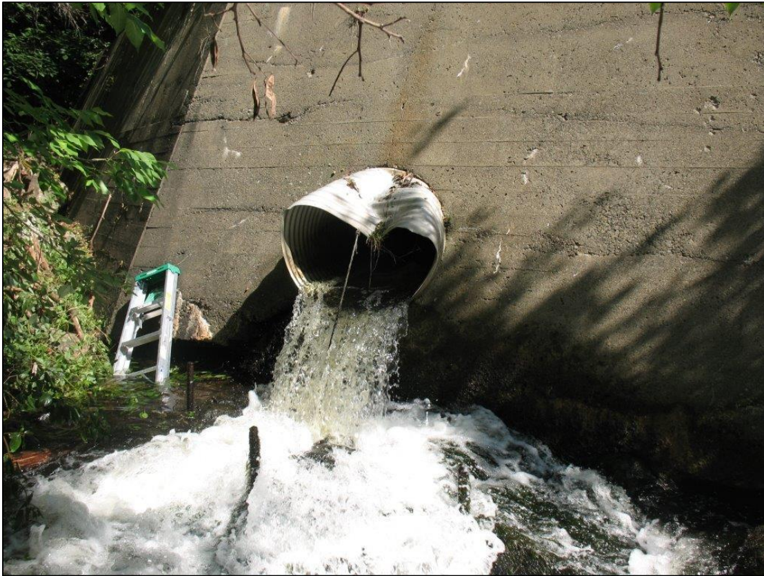
Photo 17. Leakage Discharge from Right Outlet Culvert.
