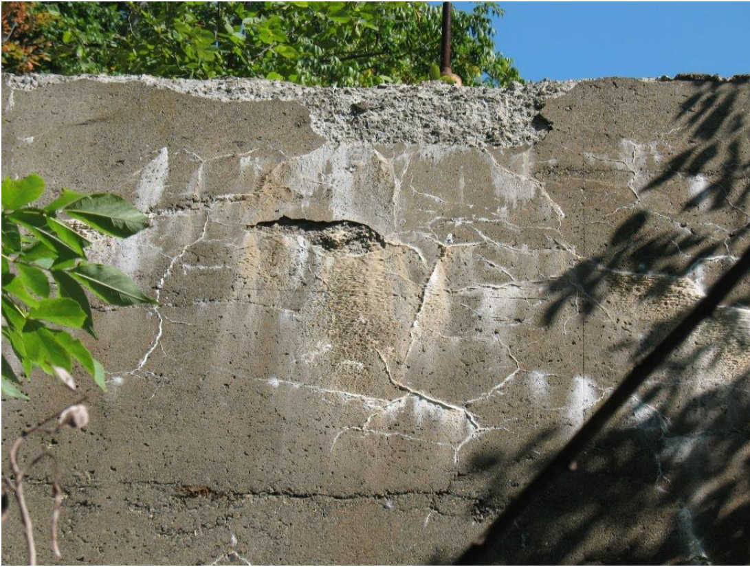
Photo 11. Right Nonoverflow Structure: Upstream Face Concrete Spalling and Deterioration.
