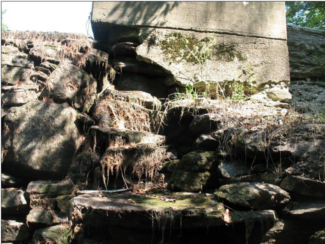
Photo 6. Downstream Face of Left Spillway Pier: Cavity and Base Undermining.
