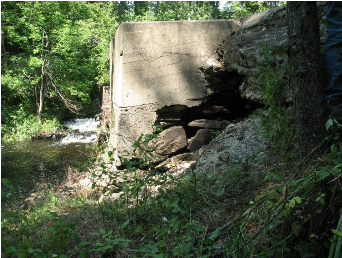
Photo 7. Left Spillway Pier Landside Large Cavity.
