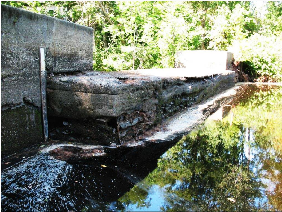
Photo 3. Upstream Face of Spillway and Left Nonoverflow: Note Voids and Deep Deterioration.
