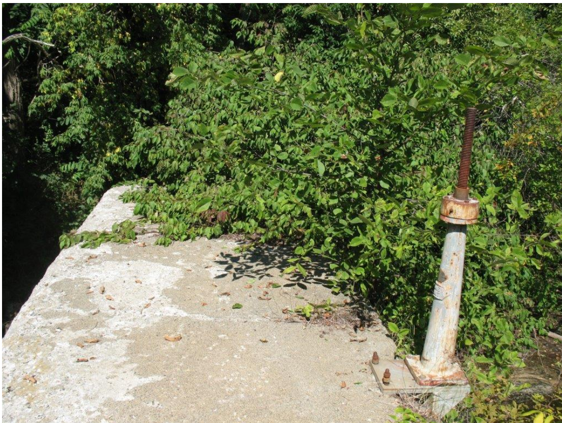
Photo 10. Top of Right Nonoverflow at Right Outlet Gate Operator: Note Heavy Overgrowth.
