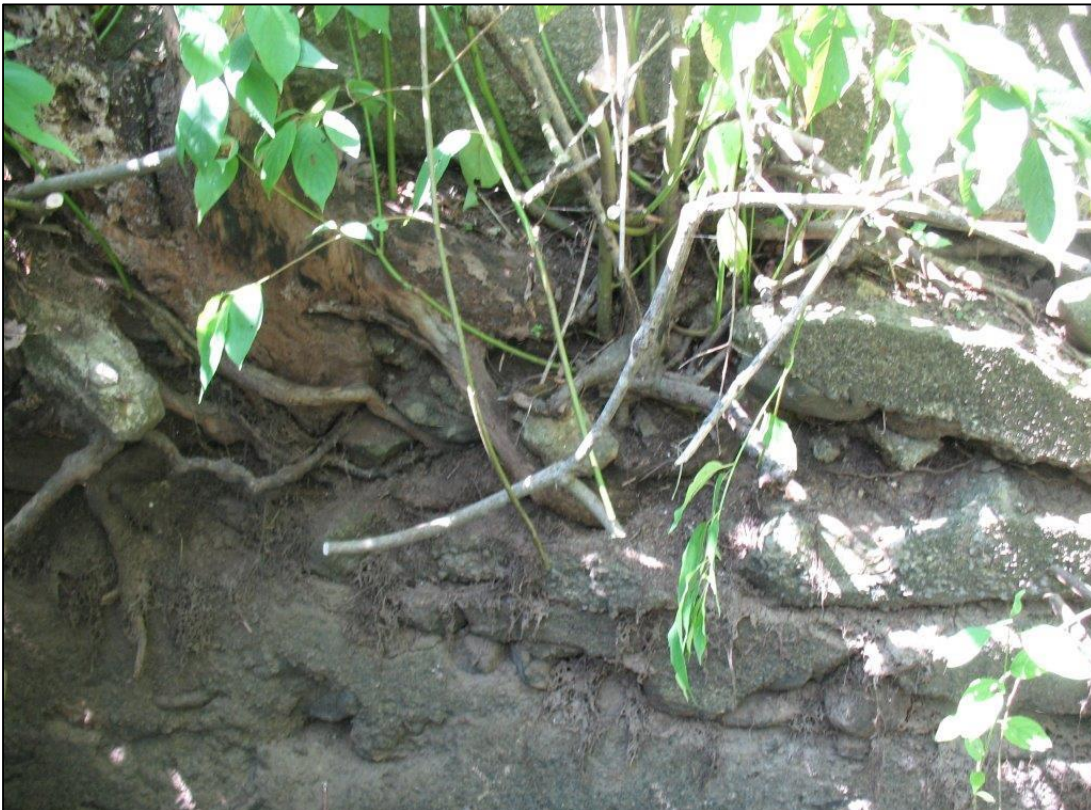
Photo 12. Right Nonoverflow Upstream Face: Masonry Rubble Uplifted by Vegetative Roots.
