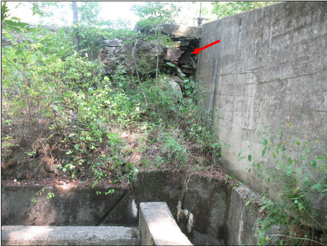
Photo 9. Left Nonoverflow: Large Cavity in Masonry Block Adjacent to Fishway (Arrow).
