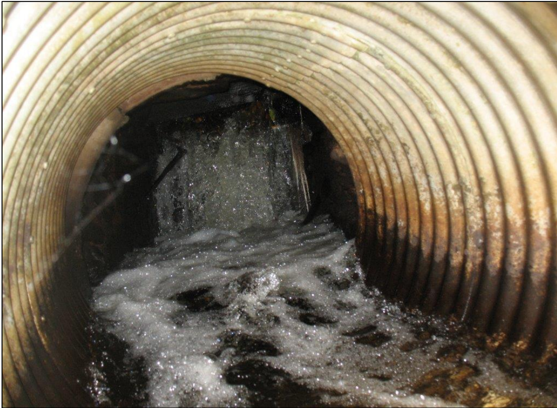
Photo 16. Leaking Gate of Right Outlet.
